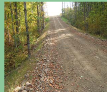
Prompt revegetation of roadsides helps to reduce the potential for sediment transfer from newly built road.
