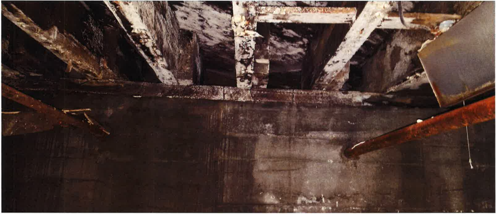
Moisture Damage and Moulds on Floor Joists (Typical)
